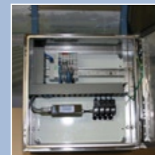
LEFT: Smart Wine micro oxygenation control panel.
