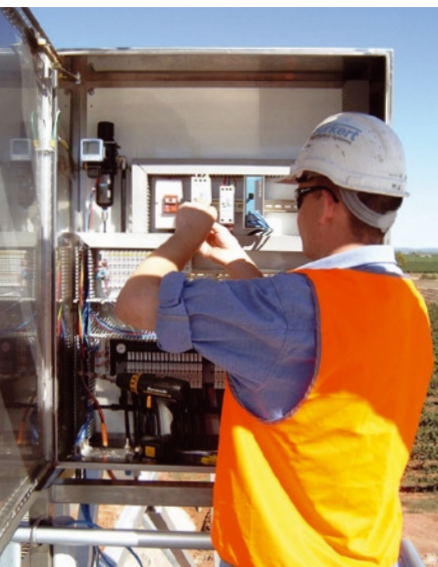
Bürkert tradesman Nelson Chymiak, commissioning an Ethernet based remote I/O system at one of Australia's largest Wineries.
